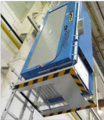
Service lift (NCV/CCV)
