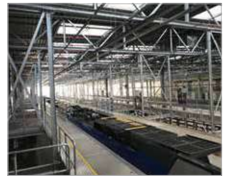
Roof work scaffolding with approx. 600m length including material lifts, cranes and PPE
