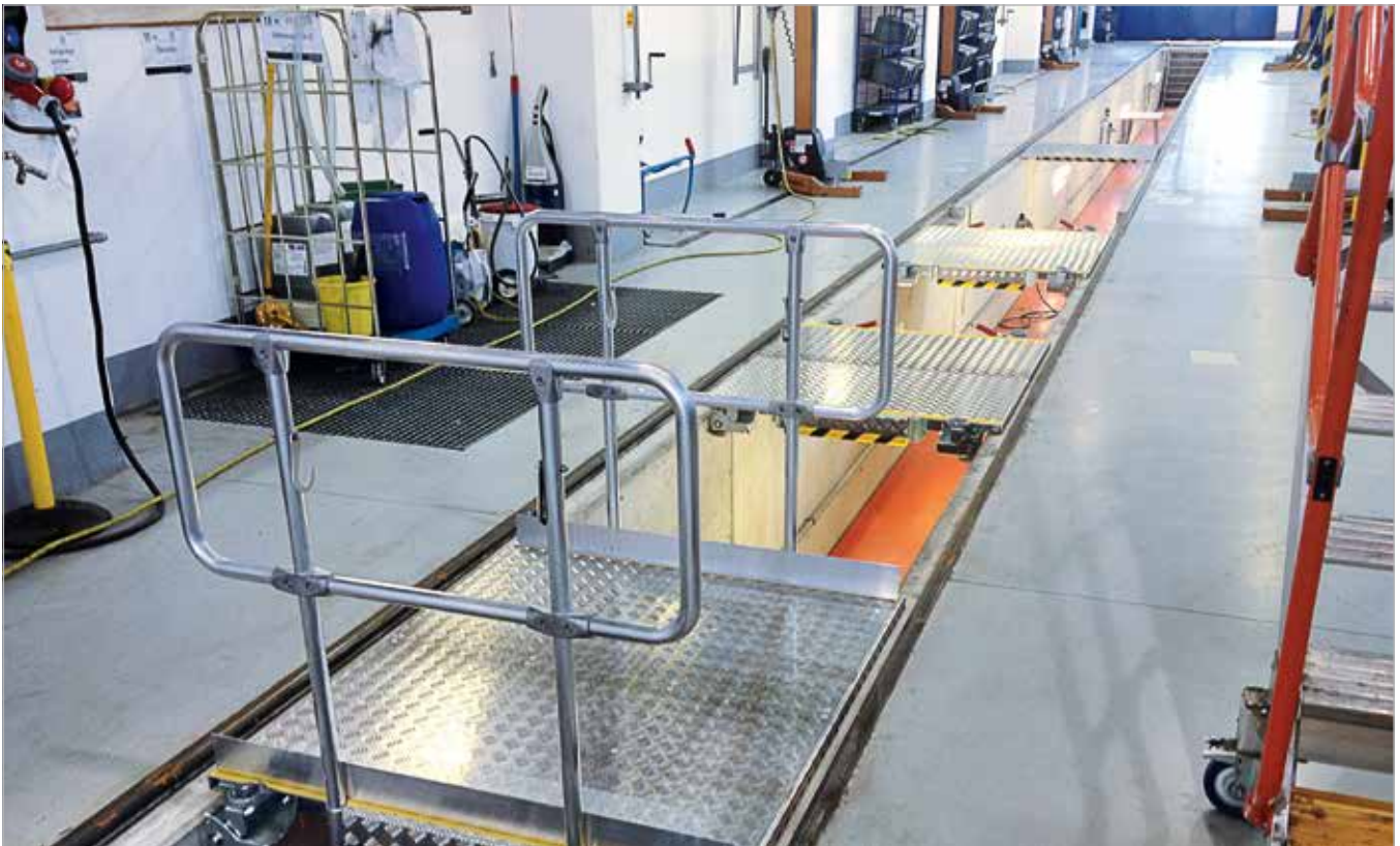
Mobile rail pit boards
