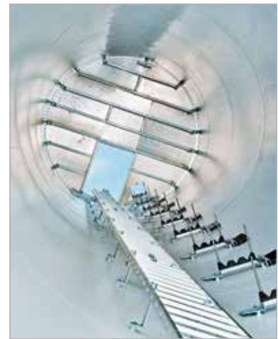
Access ladder and platform
